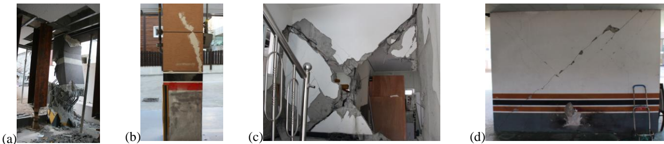
Figure 3. Examples of damaged structural members in 15 Nov. 2017 Pohang earthquake: (a) “Severe” damaged column, (b) “Medium” damaged column, (c) “Severe” damaged wall, (d) “Medium” damaged wall.
